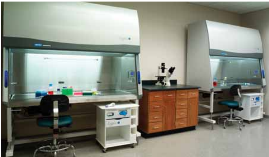
Logic Carts are shown stored beneath two 6' Purifier Logic Biosafety Cabinets on Hydraulic Lift Base Stands.
